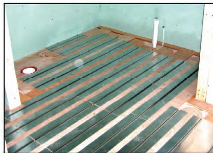
Aluminum heat transfer plates installed over plywood sleepers prior to tubing and cover sheet.
