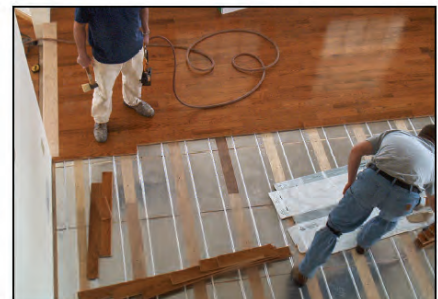
Hardwood flooring installed over tube & plate system. Note nailing areas between plates
